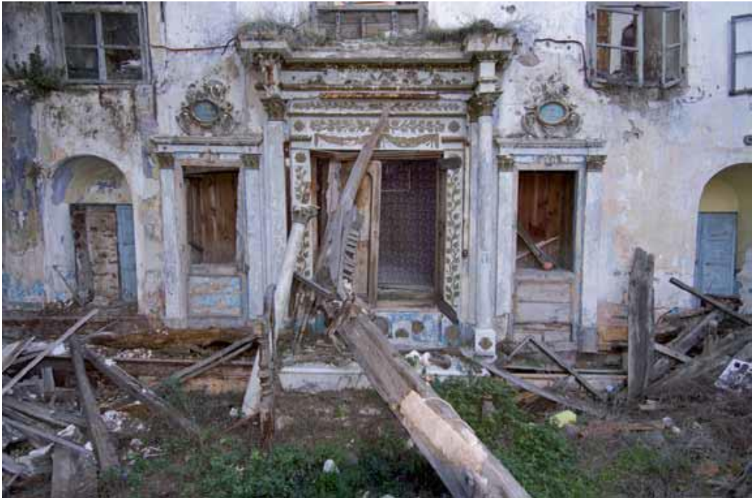
Hevra Synagogue after it collapsed
