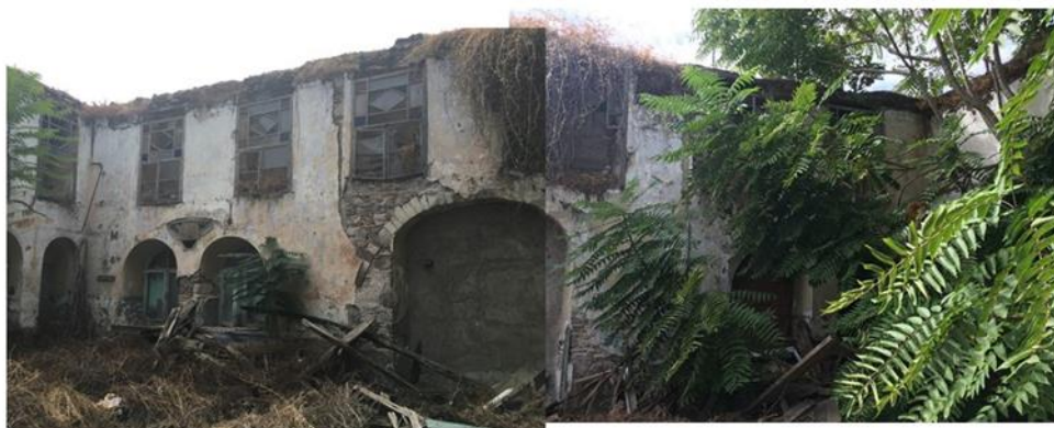
Southern elevation which includes a deep niche which may have served as another entrance to the synagogue, the remains of entries with stained glass windows and original shutters, wall decorations include paintings, wood and drywall decorations.
